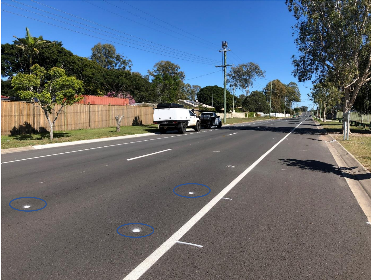
Marked pressure cell locations
