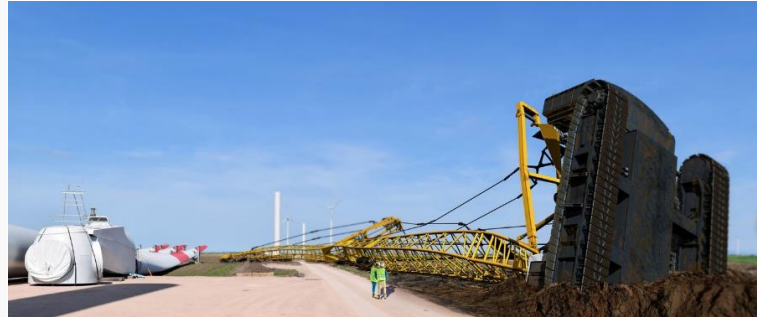
Punching shear failure
