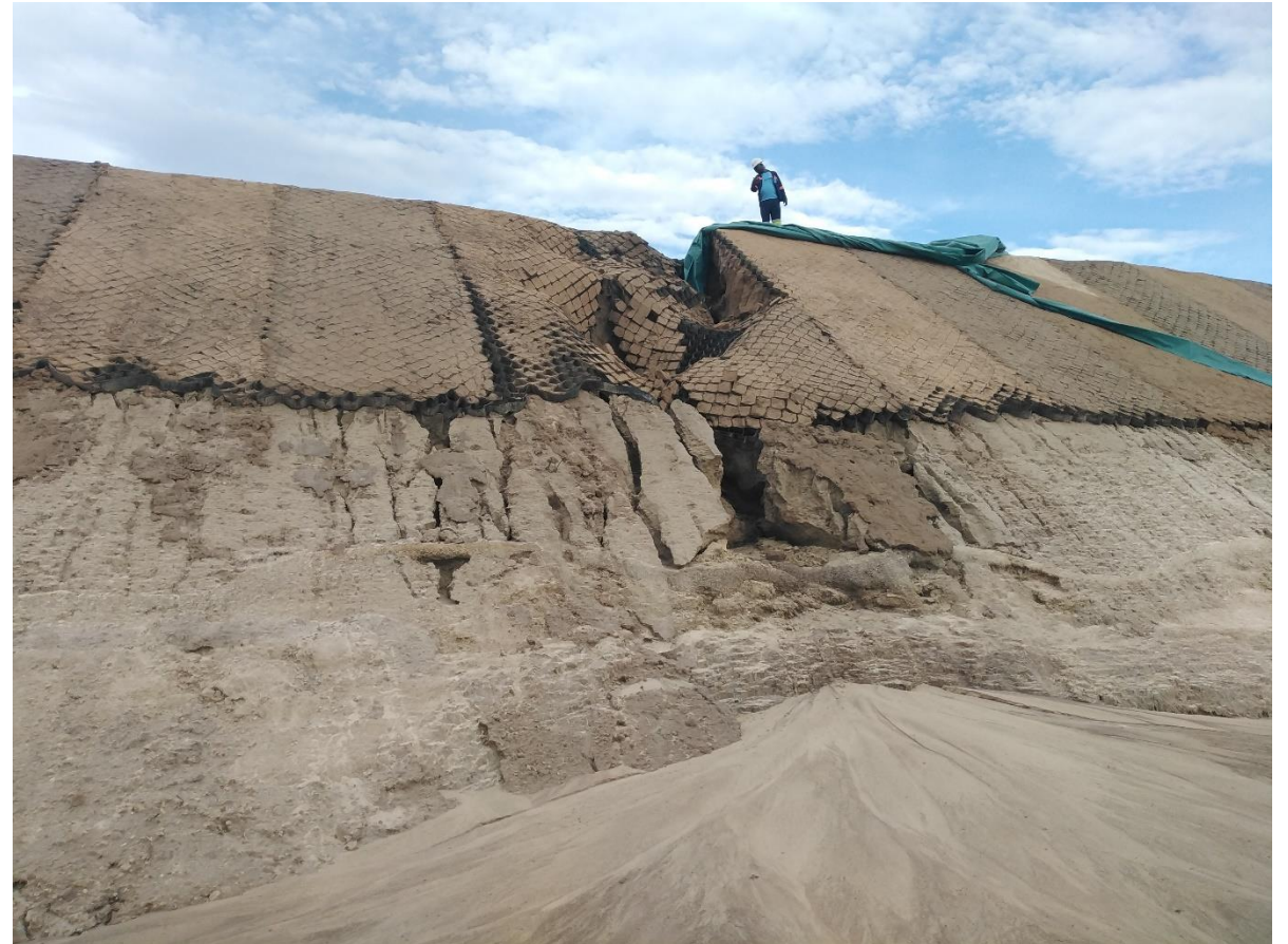
Rain damage during construction
